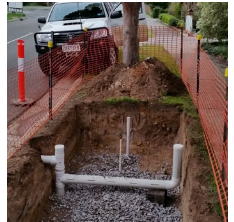
Constructing a system to irrigate street trees with stormwater generated by roads.
