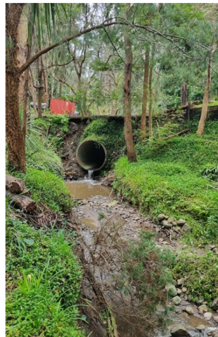
Stormwater outfall influencing a stream's physical form in eastern Melbourne.
