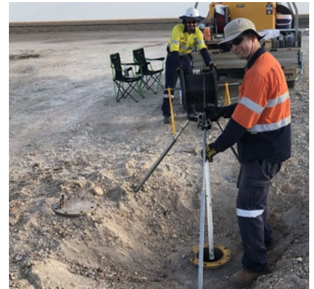
CSIRO colleagues installing a fibre-optic cable in a bore drilled by Geoscience Australia in the Northern Territory in December 2020. The cable will allow measurements of temperature and thermal conductivity to 500m depth to investigate crustal heat, aquifer properties and atmospheric temperature changes.
